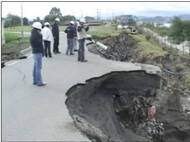
Figure 59: An example of damaged water transmission pipelines in the 2010 Chile earthquake. This limited water availability for emergency response as well as for businesses and daily living. (Technical Council on Lifeline Earthquake Engineering - TCLEE, 2010)
