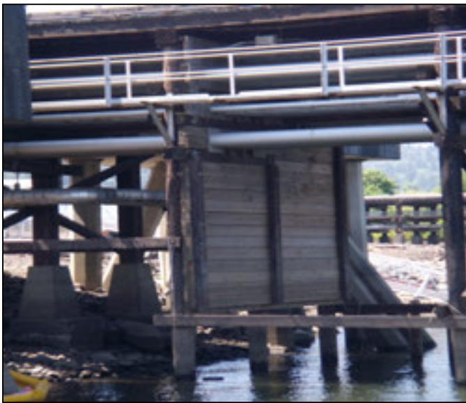
Figure 43: “Hard point” fixity of petroleum pipeline is located under this pier in the CEI Hub and is considered to be seismically vulnerable. (DOGAMI photo)
