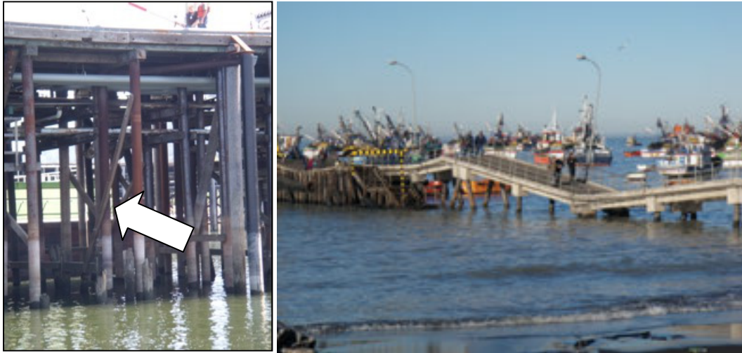
Left: Lateral timber bracing for steel plumb piles in the CEI Hub is considered inadequate by California's MOTEMS standards. (DOGAMI photo) Right: An example of a damaged pier in the 2010 Chile earthquake (Technical Council on Lifeline Earthquake Engineering – TCLEE, 2010)
