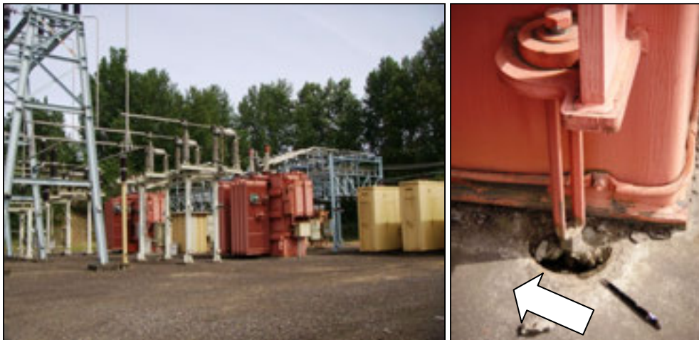
Figures 68 and 69: The photo on the left shows high voltage transformers (orange color) in the CEI Hub that require proper anchorage. The close-up photo on the right shows that the transformer is anchored, but the anchorage was poorly installed or poorly maintained as evidenced by the amount of grout that is missing. (DOGAMI photos)
