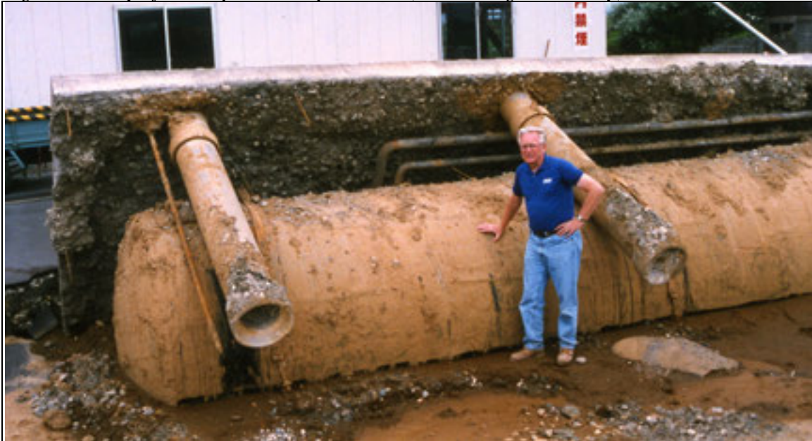
Figure 18: Buried tank in liquefied soil that was uplifted due to buoyancy forces in the 1993 Hokkaido-Nansei-Oki Earthquake and Tsunami in Japan (Photo permission on 1/9/12 from Youd; Youd, T.L. et al 1995, Photo taken by R. Chung)
