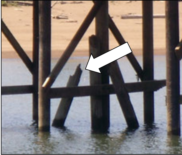
Figure 42: This pier in the CEI Hub appears to be poorly maintained with broken timber piles adjacent to working components of the pier. (DOGAMI photo)
