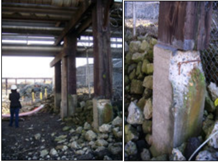
Figures 39 and 40: The close-up photo on the right shows poor timber-to-concrete connection, broken concrete and exposed rebar. Energy sector companies should maintain and upgrade infrastructure to current standards in order to protect assets and limit down-time following an earthquake. (DOGAMI photos)
