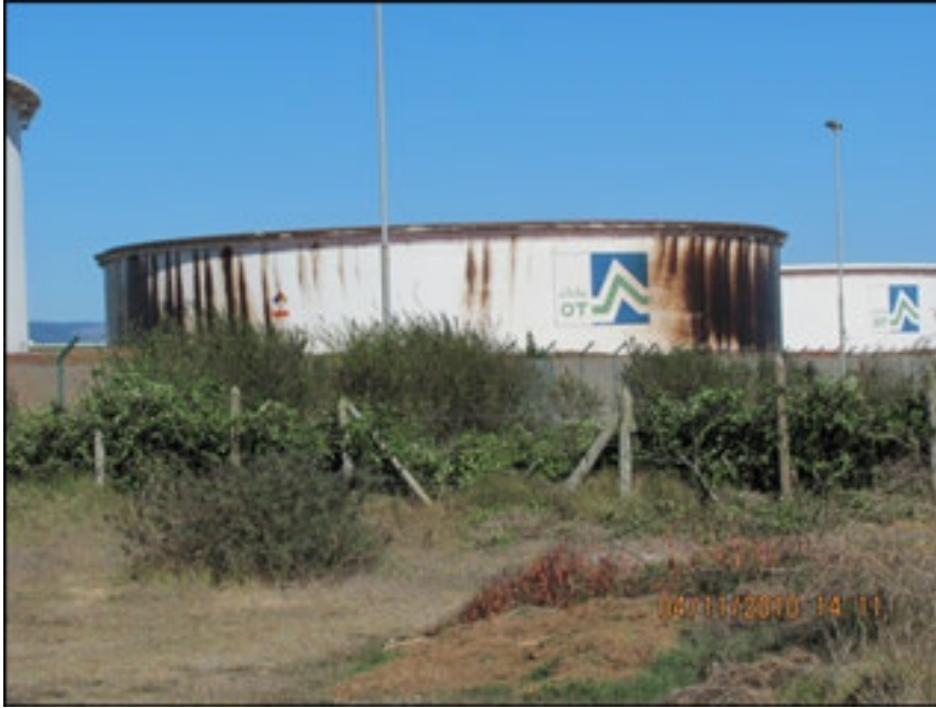
Figure 27: Sloshing of crude oil during the 2010 Chile earthquake. Note the black oil stains on the outside of the fuel tank. (Wang photo)
