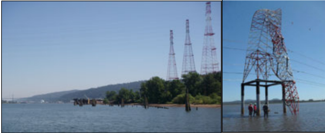
Left: These high voltage electrical transmission towers are built on a river bank in the CEI Hub susceptible to lateral spreading. (DOGAMI photo) Right: Structural damage to a high voltage transmission tower located at a river crossing in 2010 Chile earthquake (Technical Council on Lifeline Earthquake Engineering – TCLEE)
