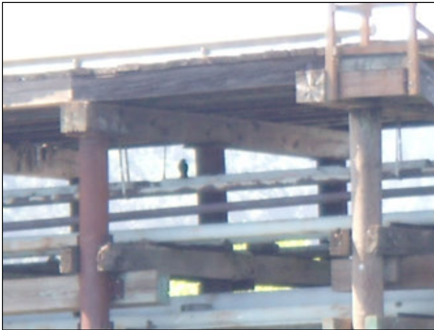
Figure 38: This photo shows generally poor condition of transverse beams supporting petroleum pipelines and cap beam in the CEI Hub. Notice the clockwise rotation of the pile cap beam in the center of the photo. (DOGAMI photo)
