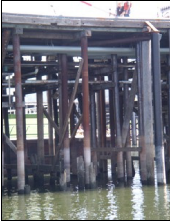
Figure 35: Lateral timber bracing for steel plumb piles in the CEI Hub is considered inadequate by California's MOTEMS standards. (DOGAMI photo)
