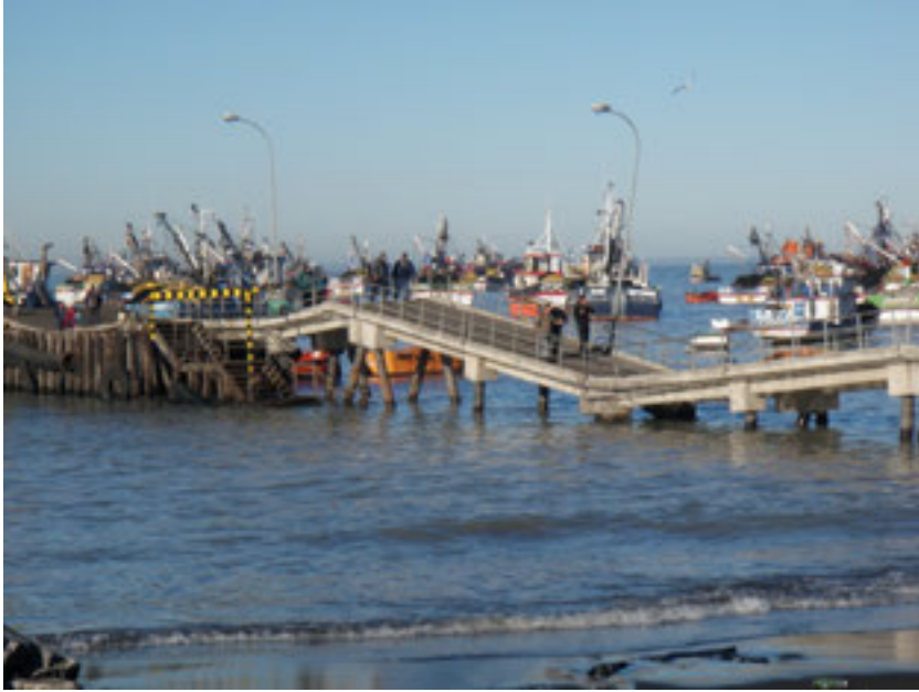
Figure 44: An example of a damaged pier in the 2010 Chile earthquake (Technical Council on Lifeline Earthquake Engineering – TCLEE - 2010)
