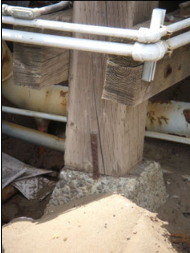
Figure 36: This under-designed foundation in part of an oil terminal pier in the CEI Hub is considered inadequate. Based on previous regional studies, boring logs from an adjacent facility, and on-site visual inspection of the surficial soils, this area has high susceptibility for liquefaction and lateral spreading. (DOGAMI photo)
