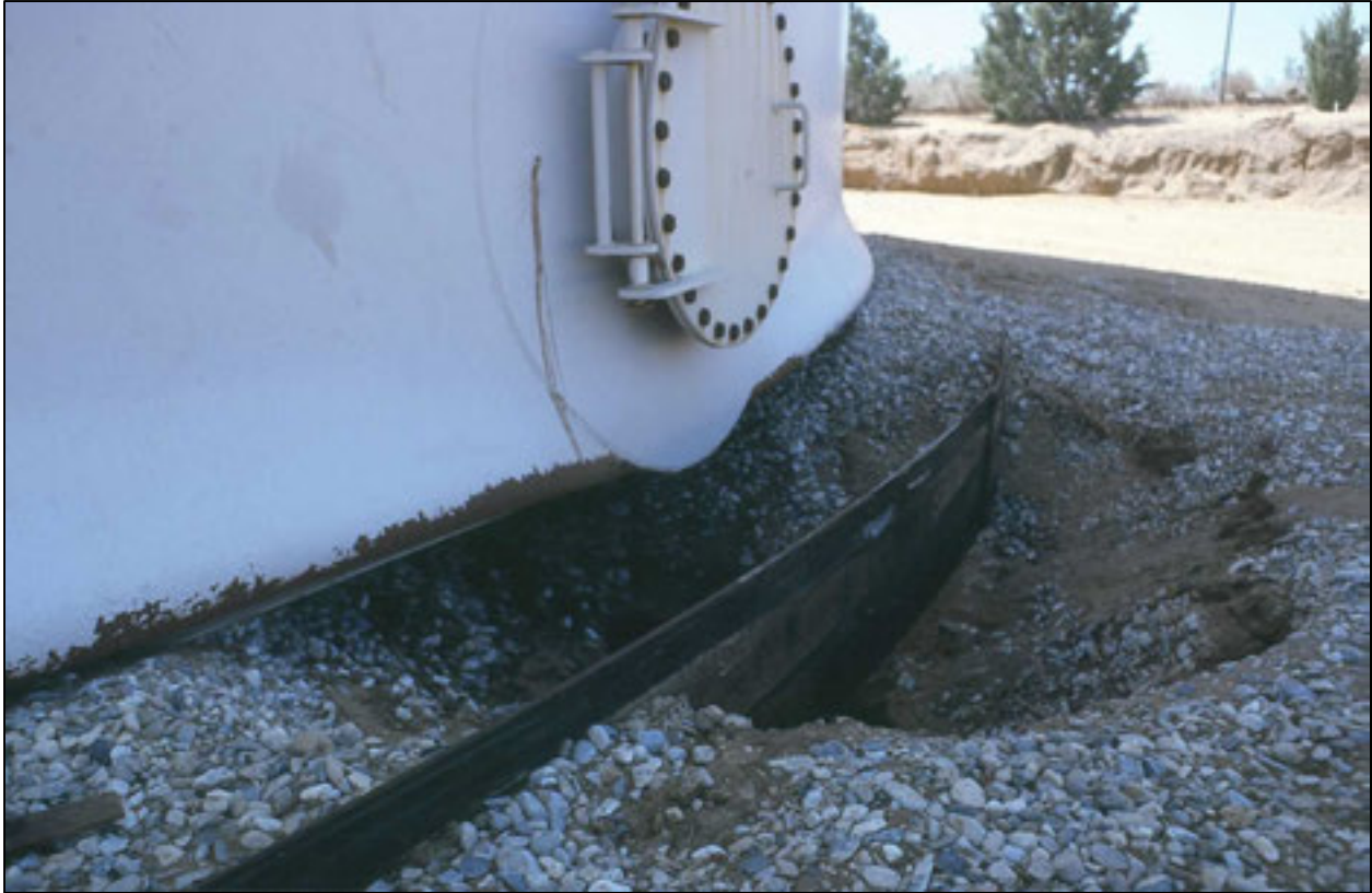
Figure 26: Welded steel water tank damaged in 1992 Landers, California earthquake. (Photo - Curt Edwards, Technical Council on Lifeline Earthquake Engineering - TCLEE)
