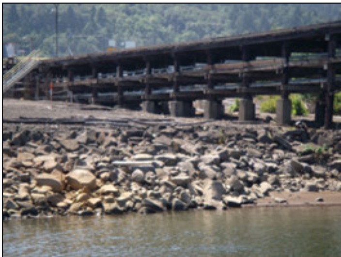
Figure 37: The area by this pier in the CEI Hub is used to transport liquid fuel. Based on previous regional studies, boring logs from an adjacent facility, and on-site visual inspection of the surficial soils, this area has high susceptibility for liquefaction and lateral spreading. (DOGAMI photo)
