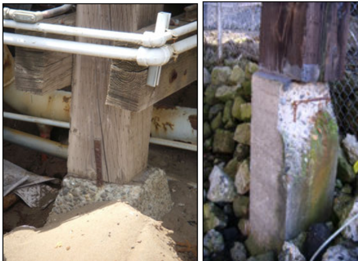
This under-designed oil terminal pier foundation (left) in area with high susceptibility for liquefaction and lateral spreading in the CEI Hub and the poor timber-to-concrete oil terminal pier connection and exposed rebar foundation (right) in the CEI Hub are considered inadequate. (DOGAMI photo)
