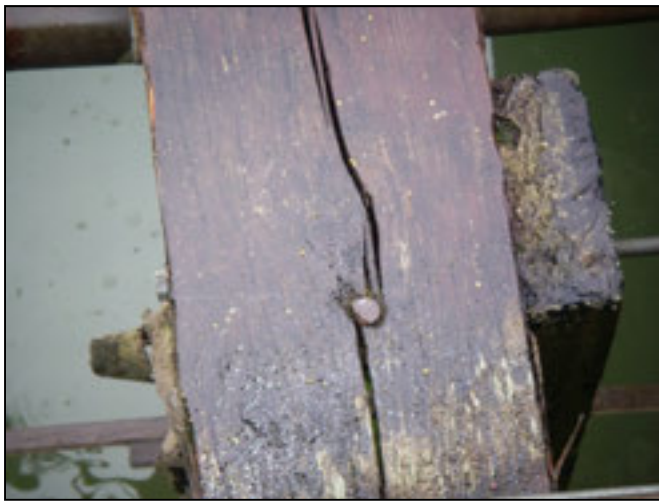
Figure 41: The connection on this pier in the CEI Hub appears to have deteriorated due to a split in the timber beam. This type of damage suggests that the condition of the structure may not be routinely monitored and maintained and that the overall pier is seismically vulnerable. (DOGAMI photo)
