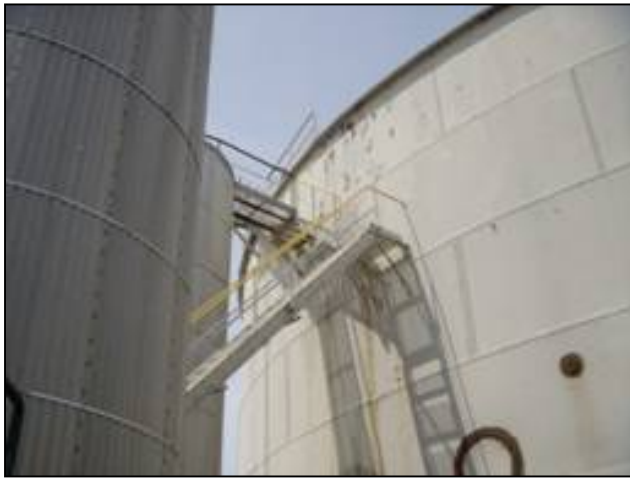
Figure 63: The elements connecting the tops of these two tanks in the CEI Hub may cause damage to the tanks during shaking due to differential displacements. (DOGAMI photo)
