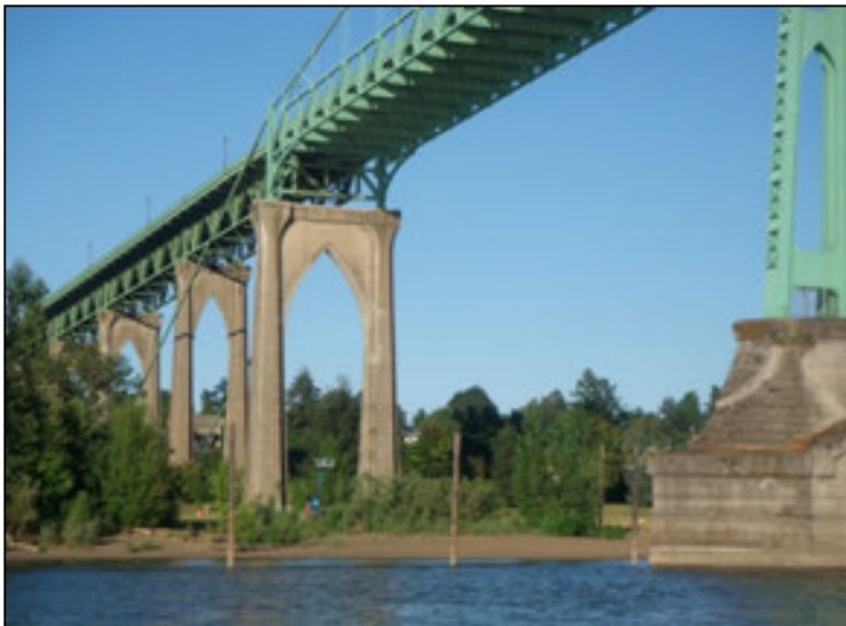
Figure 55: The 1931 St. Johns Bridge crosses the Willamette River in the CEI Hub. The tall columns that are part of the approach are seismically deficient. (DOGAMI photo)
