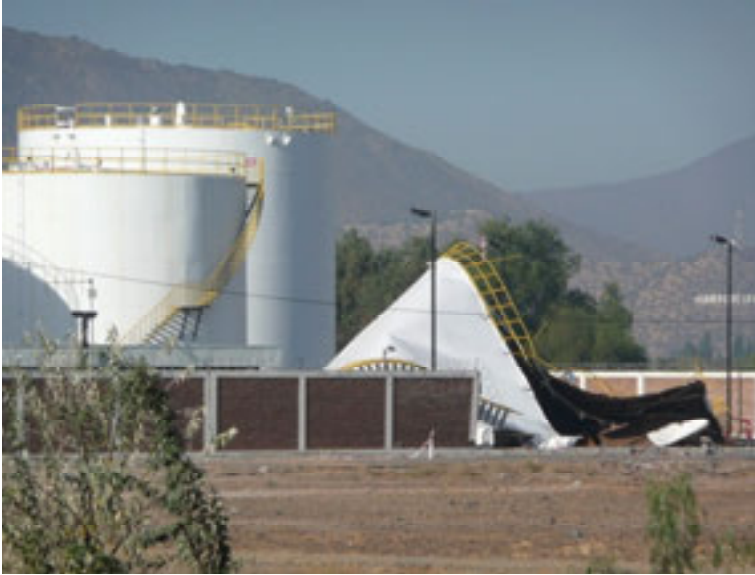
Figure 58: Structural damage to water tank located in fuel tank farm in Santiago from the 2010 Chile earthquake (Technical Council on Lifeline Earthquake Engineering - TCLEE)
